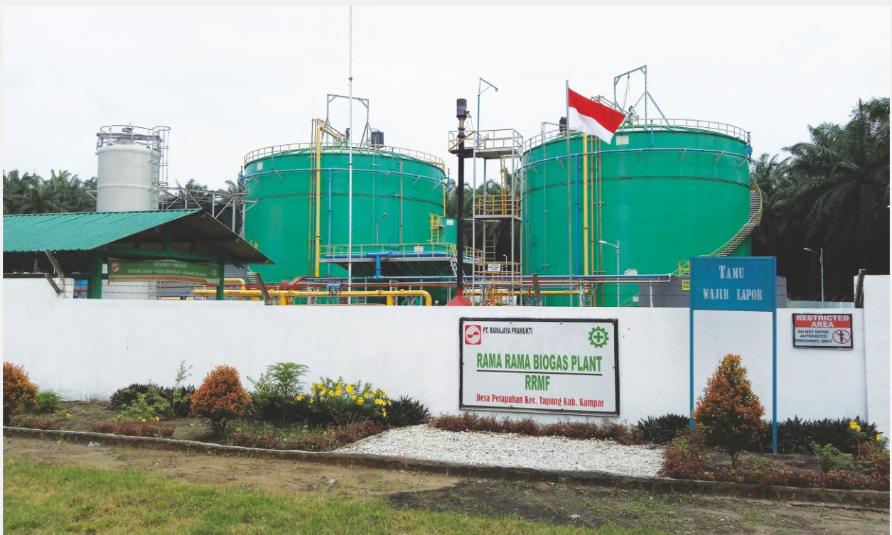
Success Story: Biogas Power Plant -1670 KW
