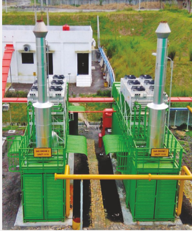
Success Story: Biogas Power Plant - 2134 KW
